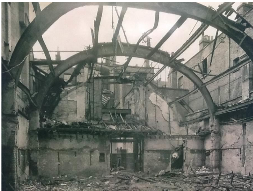
Figure 2: Bomb damage to the 1883 meeting house, 1941, looking west towards the lobby (photo supplied by Westminster Friends)
