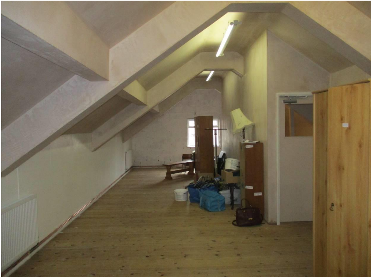
Figure 2: Loft space due to be converted into a meeting room with storage facilities.
