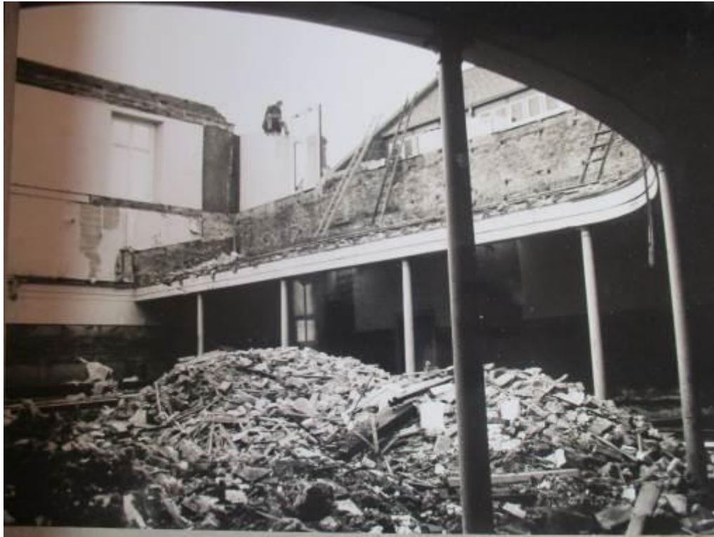
Figure 2: The former main meeting room (1817) being demolished in the 1970s (Friargate MH archive)
